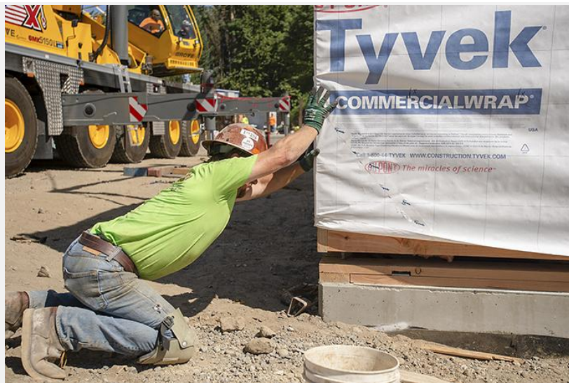
Darren Kilbourne, a laborer with Bent Level Construction, muscled a modular box into position. (Josh Kulla/DJC)
