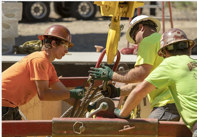
Bent Level Construction employees, from left, Brody Humphrey, Cody Humphrey, and Darren Kilbourne prepare a steel rigging frame that will be used to lift a modular box into place. (Josh Kulla/DJC)
