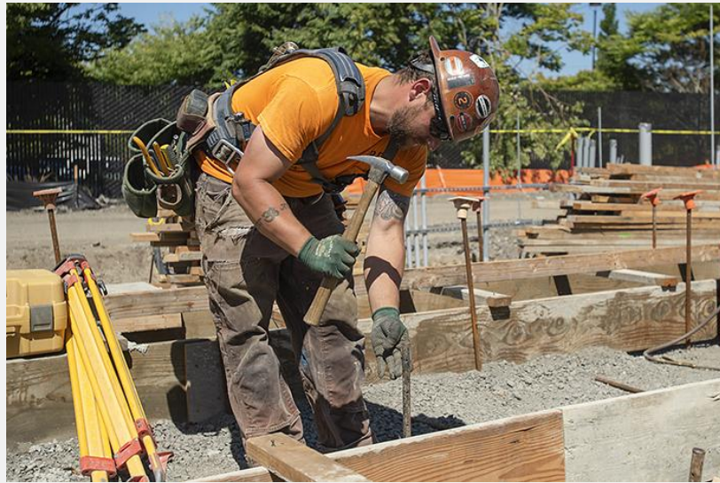
Jambavan Zakheim, a journeyman carpenter with Local 1503 and RDF Builders, constructs foundation formwork. (Josh Kulla/DJC)
