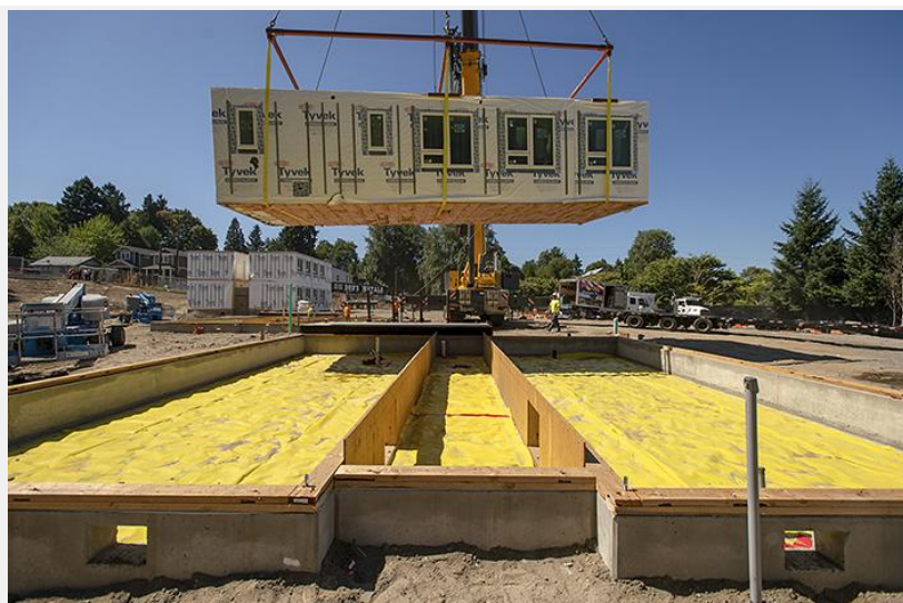
The first of four modular boxes comprising an entire building is flown into place atop a concrete foundation at the LISAH project site. (Josh Kulla/DJC)
