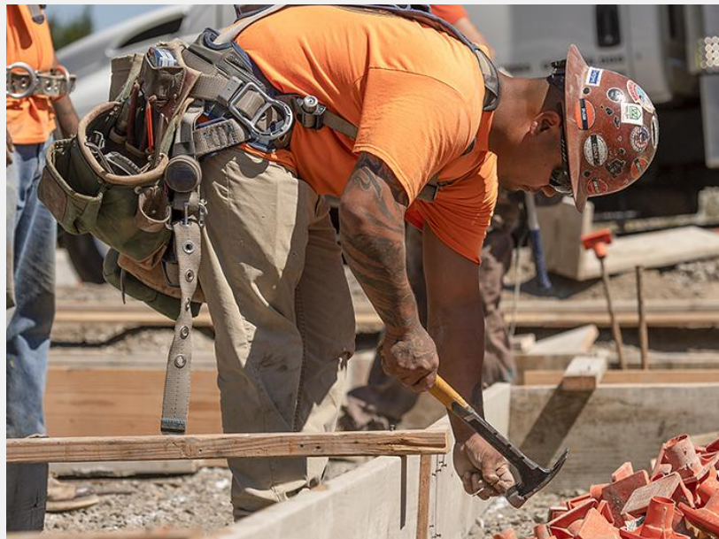
Apprentice carpenter Daniel Perez, a member of Local 1503 and an employee of RDF Builders, constructs formwork at the LISAH site. (Josh Kulla/DJC)
