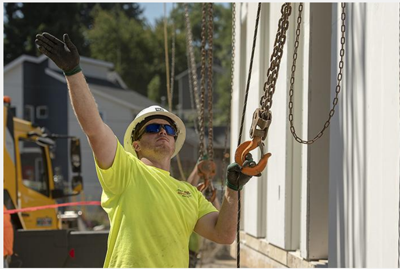
Cody Humphrey, foreman of a crew of laborers with Bent Level Construction, signals to a crane operator while rigging a modular box. (Josh Kulla/DJC)
