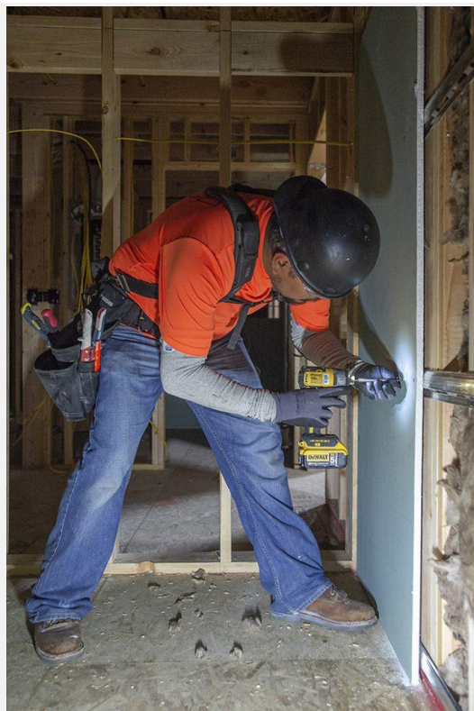
Installer Luis Rodriguez of MidValley Construction installs sheets of drywall inside a modular unit being manufactured for the LISAH project at the Mods PDX warehouse in North Portland. (Josh Kulla/DJC)
