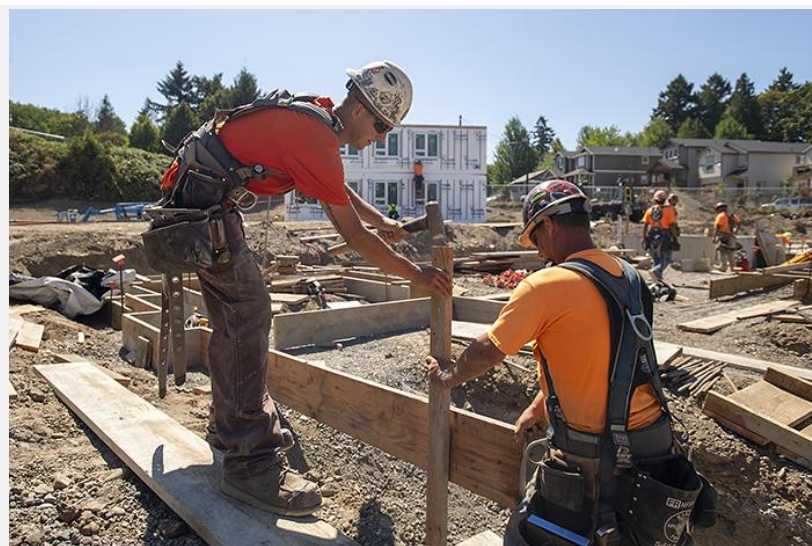
Journeyman carpenters Shane Gill, left, and Dan McHarge, both members of Local 1503 and employees of RDF Builders, construct formwork for the foundation of one of the three modular buildings at the LISAH job site. (Josh Kulla/DJC)
